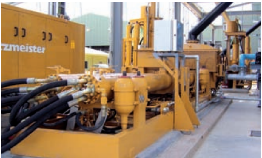
Two KOS 25100 are pumping fly and bottom ash / Kogan Creek, Australia
