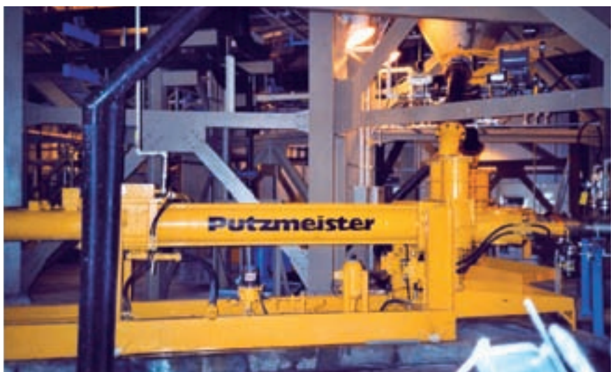
HSP 25100 fly ash pump at Colstrip power plant
